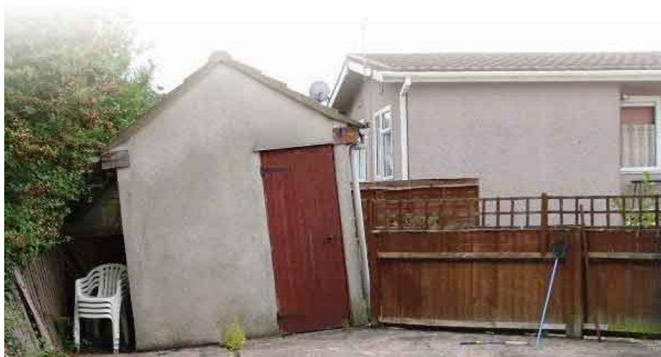
Figure 1-8: House damage due to the sinking of the foundation.
