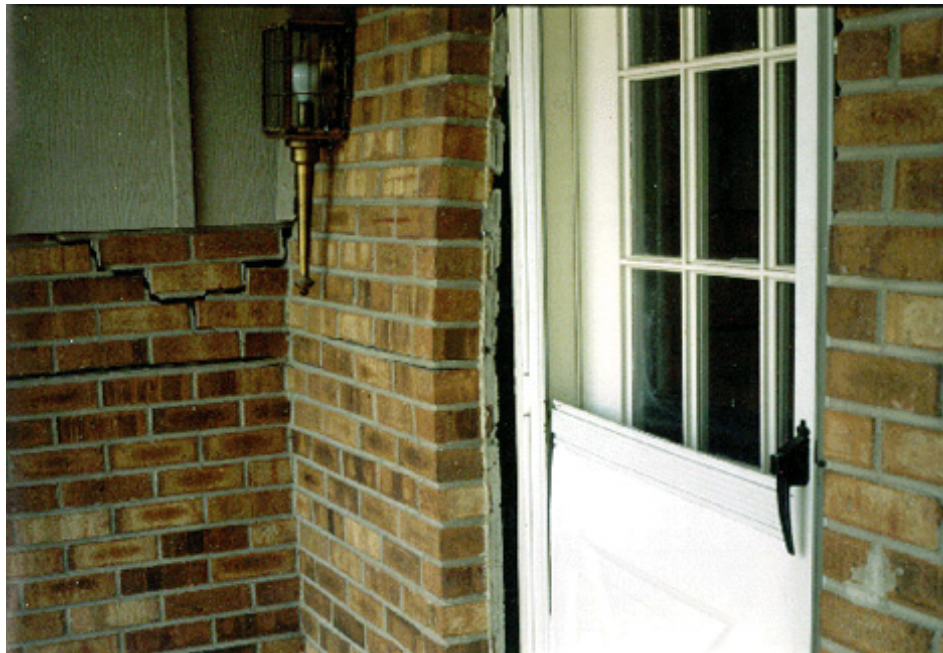
Figure 1-7: House damage due to differential heave. Photograph by David C. Noe, Colorado Geological Survey.
