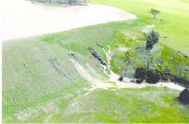
Figure I .1: Embankment degradation caused by fine particle migration ( Irons et al., 2014 )
