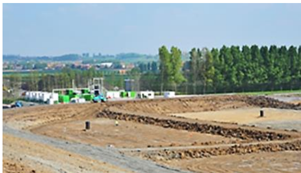
Figure 51: Storage site in Baudelet Environnement, Blaringhem, France
