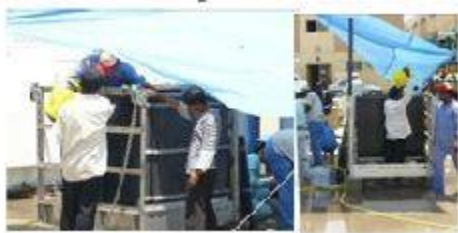
Figure 9: Protection of UF membrane.
