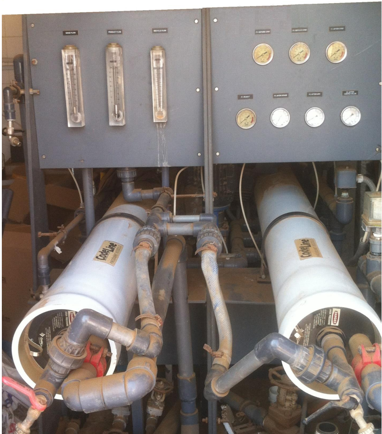
Figure 30: The membrane and chemical of the pilot unit
