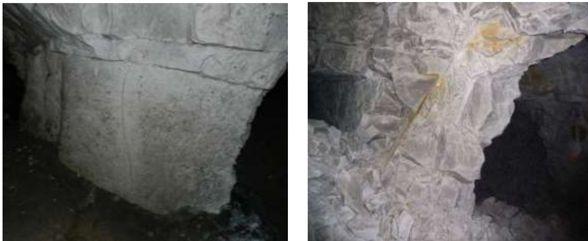
Figure 1.28. Mechanical fissures and faults at the pillars
