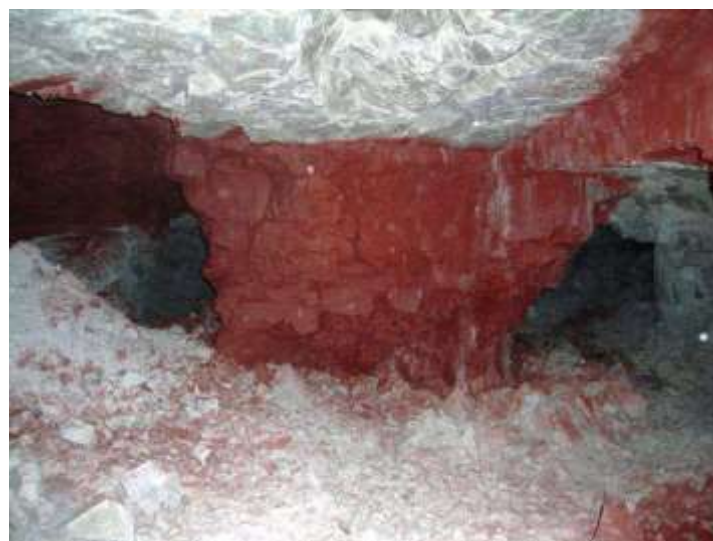
Figure 5.7. Degraded pillar in the cavity of Don Bosco in Lille on October 2011.
