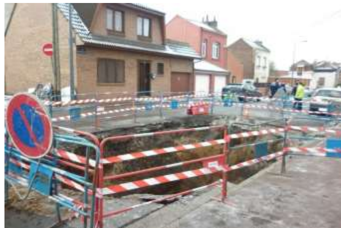
Figure 1.18. General view of the collapse above the Don Bosco cavity in Lille recorded in February 2012 (by City of Lille)
