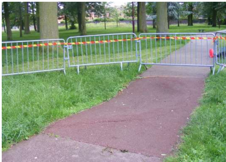
Figure 1.10. Case of generalized collapse in Lille, North France
