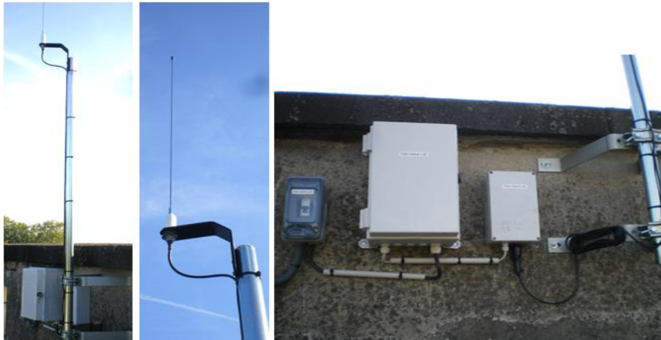
Figure 2.18: Base station on the roof of C7 building
