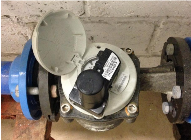
Figure 2.15: Compact transmitter installed on the water meter in the building C of the engineering school "Ecole Centrale de Lille"
