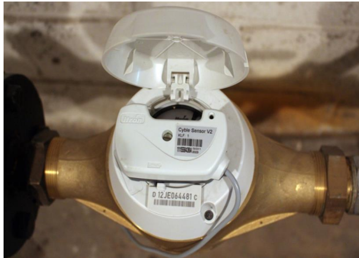
Figure 2.17: Deported transmitter installed in the SN5 building
