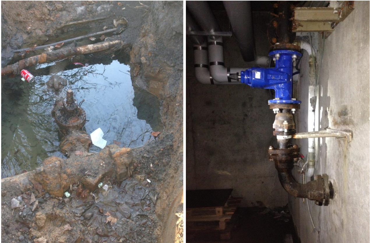
Figure 2.9: Valves in the demo site
