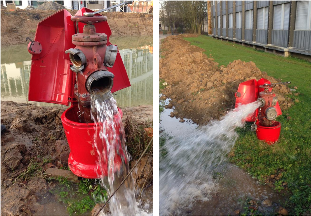
Figure 2.29: Simulated leaks using the fire hydrants
