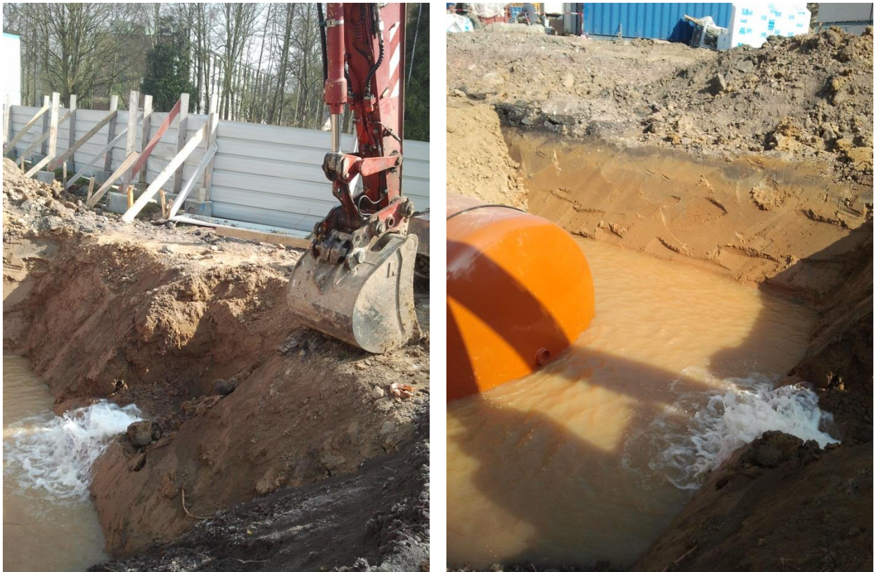
Figure 3.20: Burst pipe in the construction site of the new library (17 March 2015)
