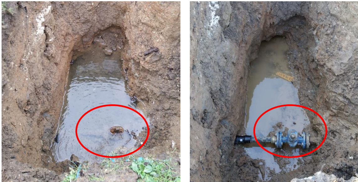
Figure 4.7: Leaking valve before and after leak repairs
