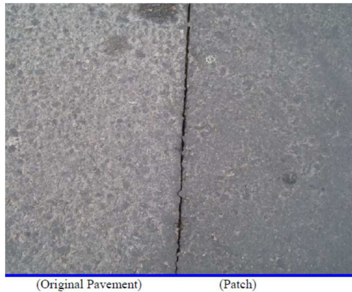
Figure 1.13 : Absence de colmatage des joints de tranchée ( Nichols Consulting Engineers 2007 )
