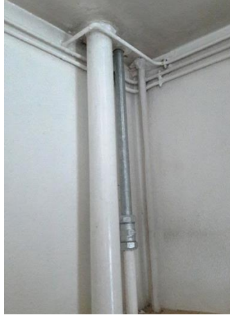
Figure 2.9 View plumbing pipes inside an apartment
