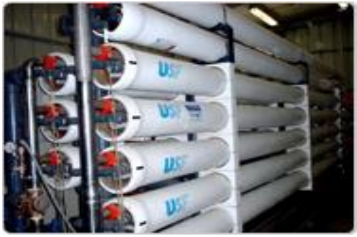
Figure 73: the water passes through semi-penetrable membranes to be desalinated. - Katsa Ashkelon company.
